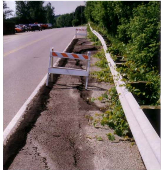
Settled Road Edge (After 3 Years)
