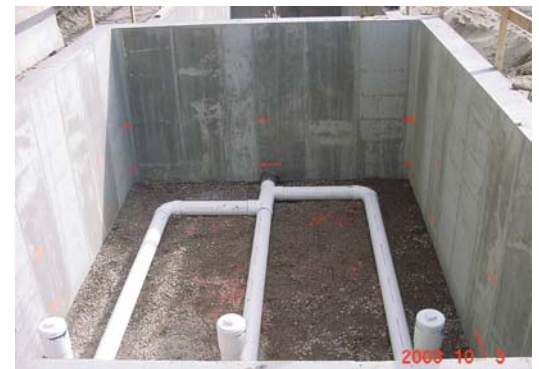
Sand Filter for Stormwater
