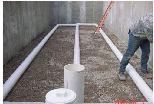
Sand Filter for Stormwater
